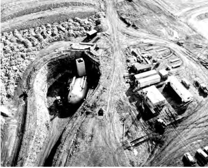
A Launch Control Facility under construction near Malmstrom AFB, Mont. Cold War requirements to build up U.S. nuclear defenses speeded up Minuteman site construction. Builders often labored year-round in three shifts, seven days a week. The Army Corps of Engineers Ballistic Missile Construction Office and its contractors built 1,000 silos between 1961 and 1966. (Image courtesy of the National Museum of the Air Force.)
